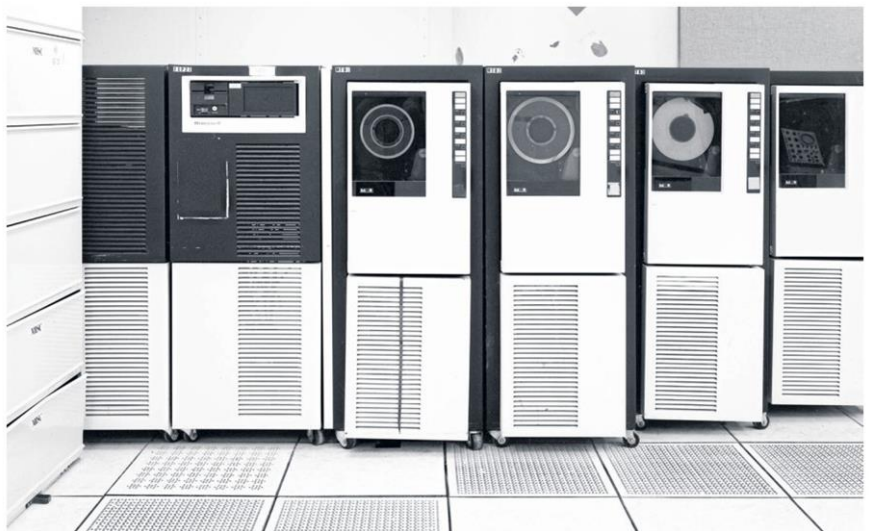
Several generations of mainframe computer systems in the bunker.
